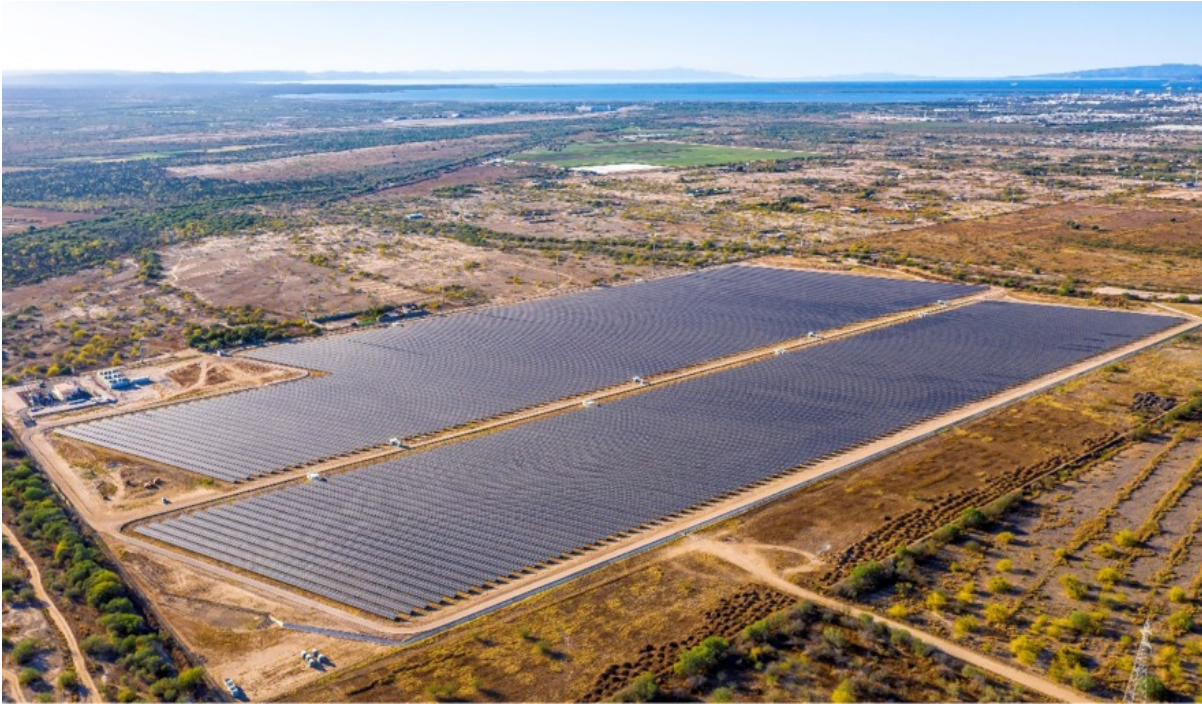
The Aura Solar III plant, La Paz, Mexico. Capacity 32MW
